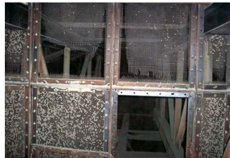
Severe LPA screen erosion
