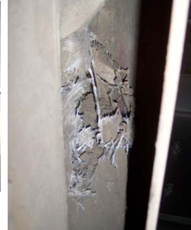
SCR reactor inlet expansion joint rupture
