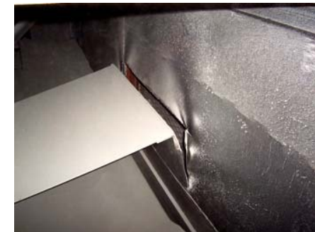
Guide vane damage to SCR outlet ductwork
