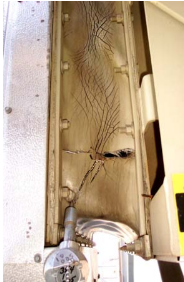
Overheated seal air expansion joint
