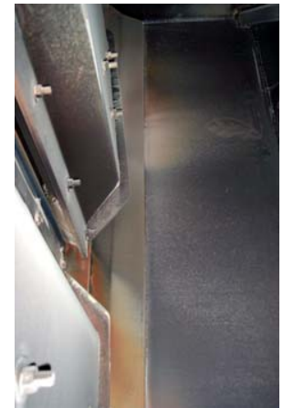
Misalignment of damper louvers
